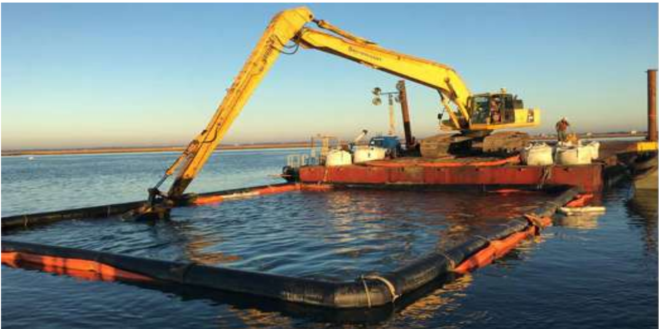
Fig.10. Suspended matter curtain around dredging area (Source: Gaia terre-bleue, Impact mer, DHI and Bird&Bird)
