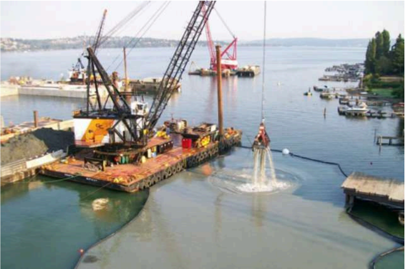
Figure 7 : Illustrations of the installation of an anti-suspended matter curtain in a dredging workshop (Web source)
