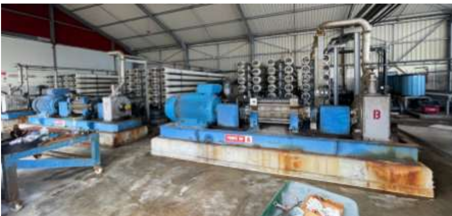
Figure 4 : The 3 reverse osmosis units (source: Gaïa, 2020)
